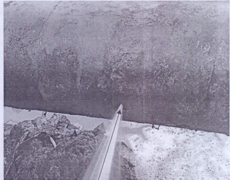
SPILL POINT (Corrosion)
